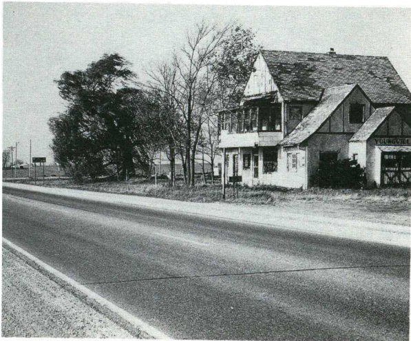
Today the Youngville Station is in an advanced state of decay. The building, however, is restorable. The original Lincoln Highway, left, stretches to the west.
